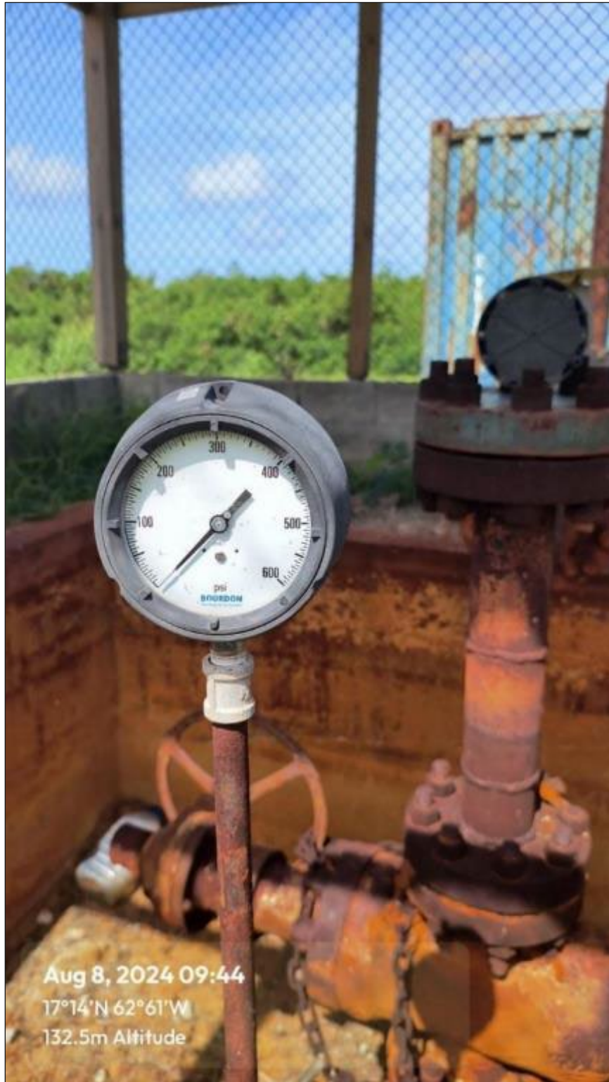
Photo 7: Pressure gauge at N-4.
